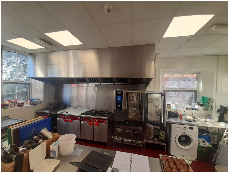
Extract hood ventilation system to shut down when fire alarm operated.
