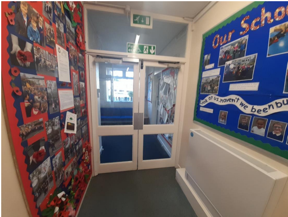
Fire doors to be replaced by new disabled access (AD Part M) compliant doors.
